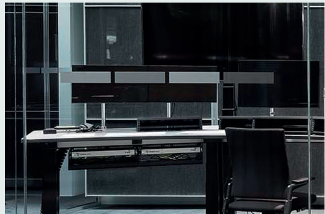
Ergonomic workstations in the SRF broadcast center: instead of bulky and noisy servers, compact extenders are located under the desks
