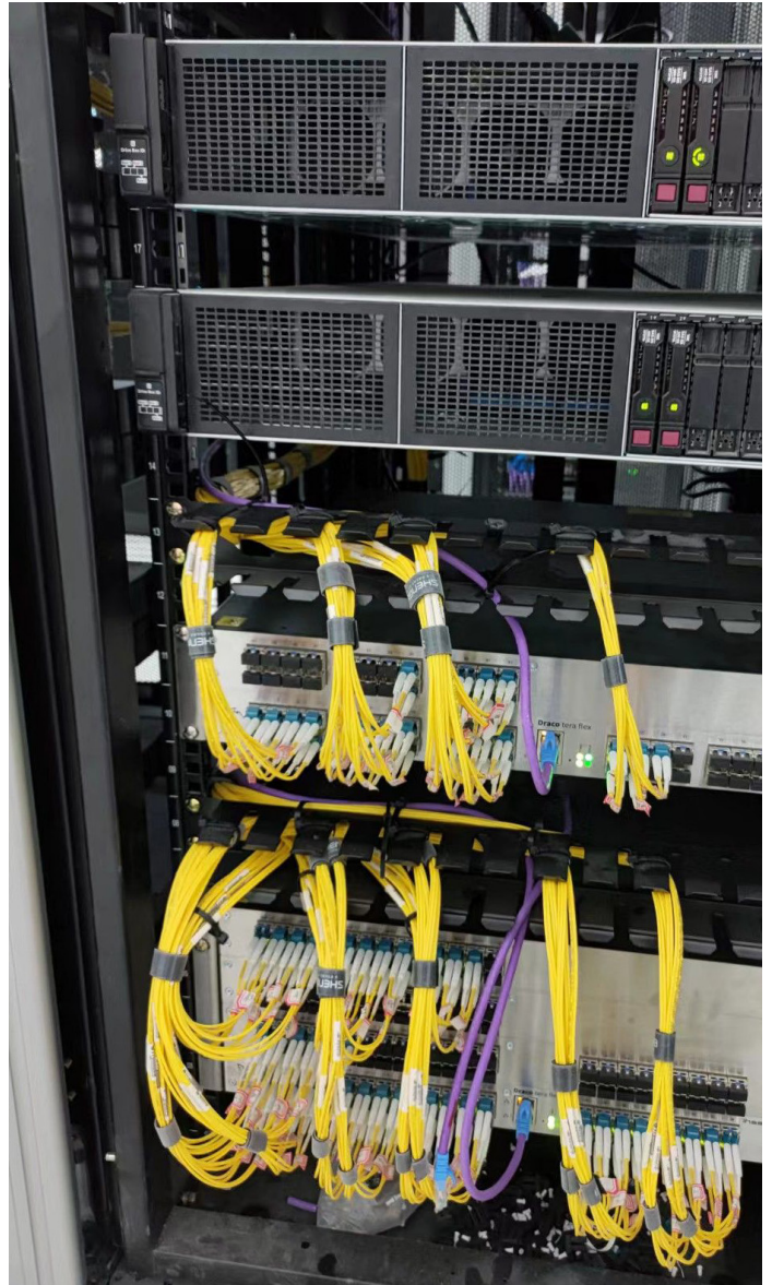
Draco tera flex matrix switches in operation
