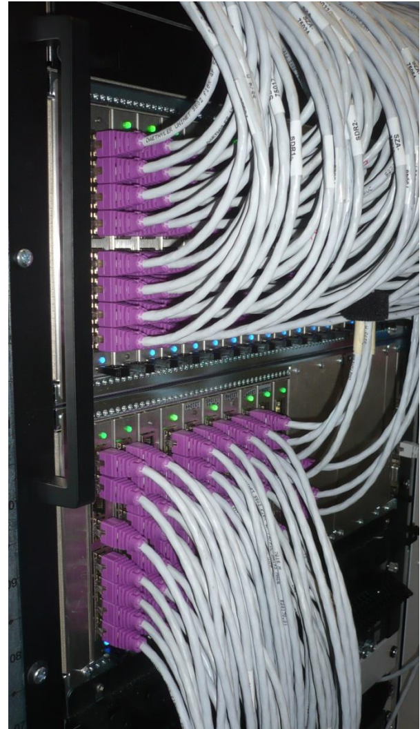
Draco tera system in operation
