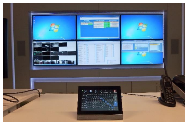
Videowall and touch screen panel in control room
